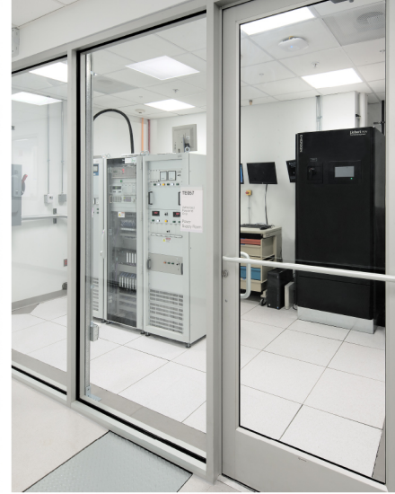
Power Supply Room
